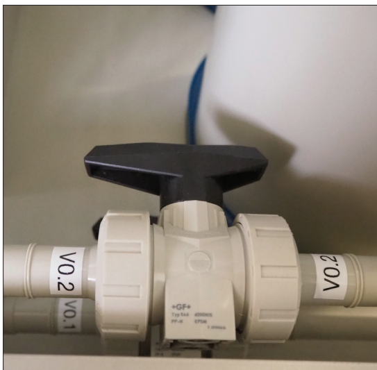
Figure 8: Open inlet valve V0.1 and V0.2
