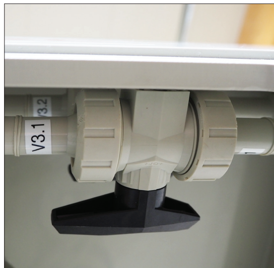
Figure 9: Open outlet valve V3.1 and V3.2
